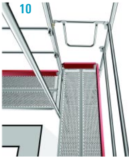
10 For a gap-free transition at the corner the frames are positioned flush.
